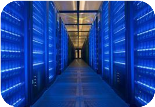
Machine room and hardware
